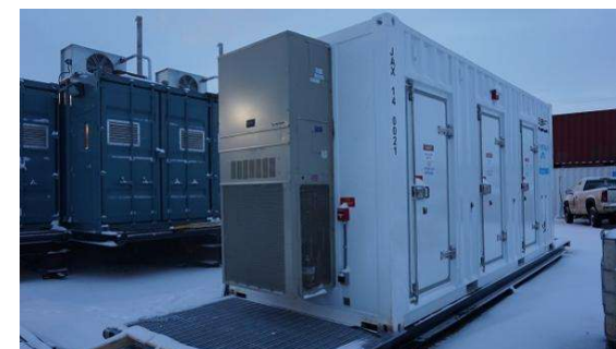
232 kWh/232 kW energy storage, © Saft
