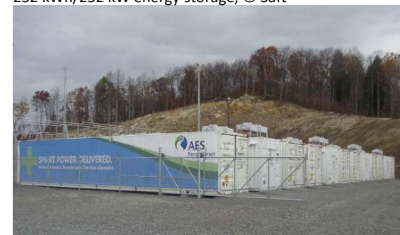
8 MWh/32 MW energy storage, © AES Energy Storage
